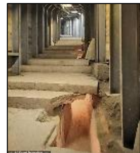
Broken road revealing drain
